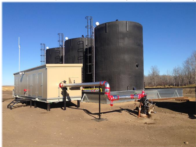
Kaisen's newly commissioned water facility (A5-29) at Edam was a key building block in nearly tripling our capacity up to 19,000 bbls of water per day
