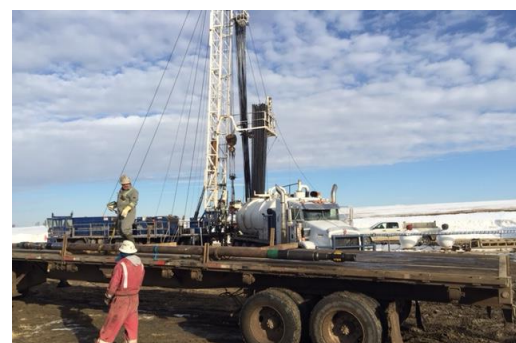
Reactivating a shut-in well acquired in a 3-section land deal in our Lone Rock area which closed in December. This well has been a great producer since its late March start-up and the acquired lands have added significant drilling inventory to the reserve book.
